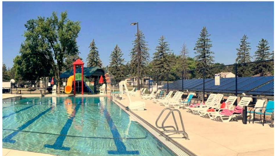
Figure 8: Parkers Prairie Pool has a thermal solar array, meaning it creates heat for the pool water. The City of Parkers Prairie is part of West Central Initiative's Municipal Solar Cohort, exploring additional solar installation to supplement the electricity that runs the water pumps.
